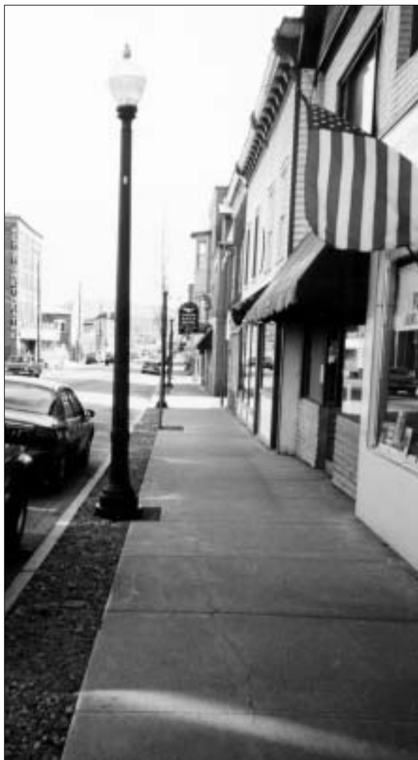
Structural soil is used to back fill the tree root/electric line trench.
